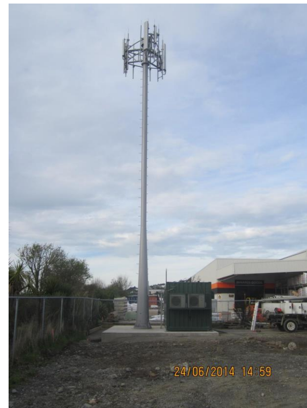
Example of LTE or 4G upgraded site in an industrial area
