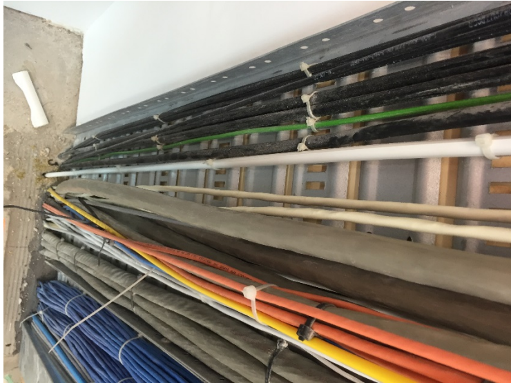
Use of existing cable trays
